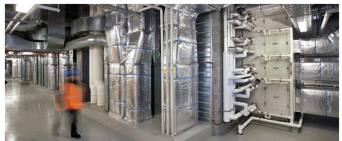
The role that HVAC systems play in fire and smoke control is a critical and often complex aspect of HVAC system design, operation, and maintenance.
